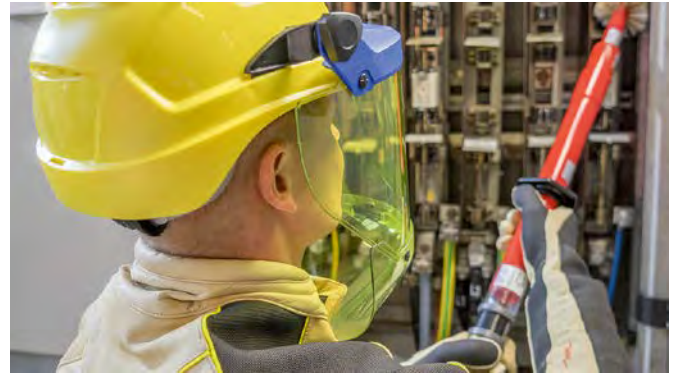
Cleaning a low-voltage switchgear using adequate personal protective equipment.
