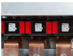
Built-in protection transformers
