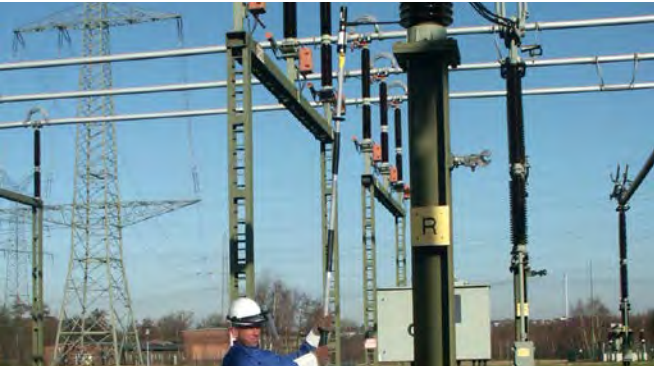
Use of an ASP distance voltage detector in an outdoor switching station
