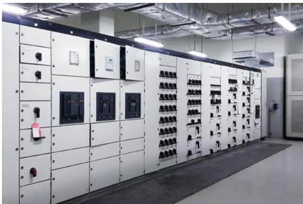
Industrial low-voltage switchgear installations
