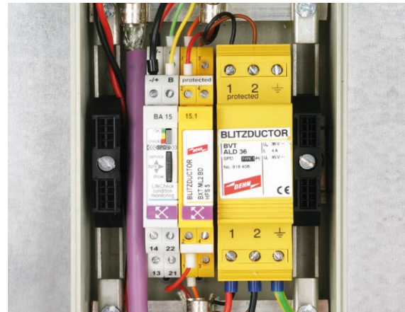
Figure 11 Protection of wind measurement equipment (anemometer)
