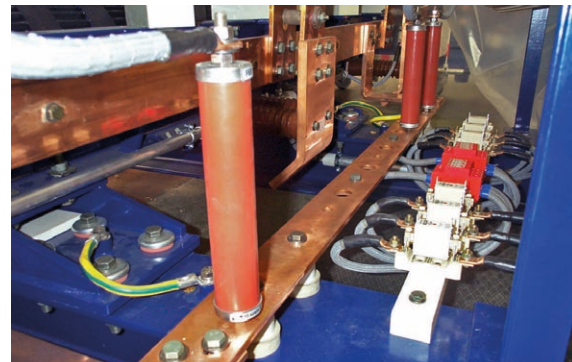
Figure 9 DEHNmid medium-voltage arresters installed in a transformer for wind turbines
