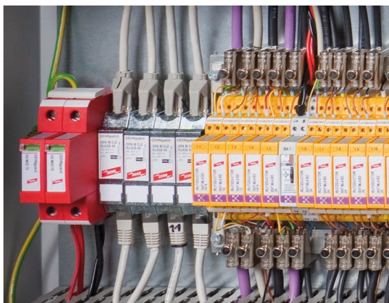
Figure 12 Example of surge protective devices in a pitch system
