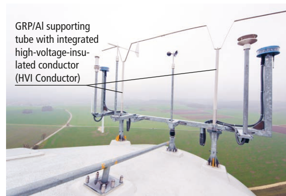
Figure 2 Example of an air-termination system for the weather station and the aircraft warning light
